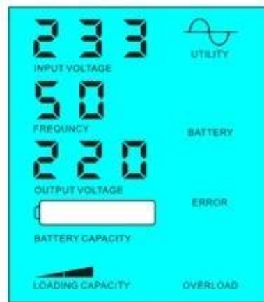
Battery dead, utility supply power
