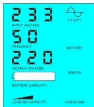
Battery dead, utility supply power
