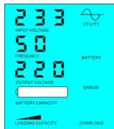
Battery unavailable, utility supply power
