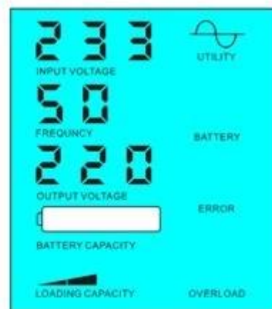
Battery dead, utility supply power
