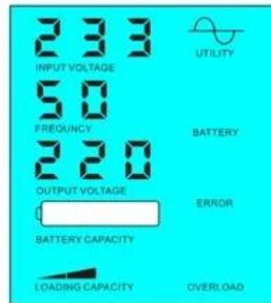
Battery dead, utility supply power
