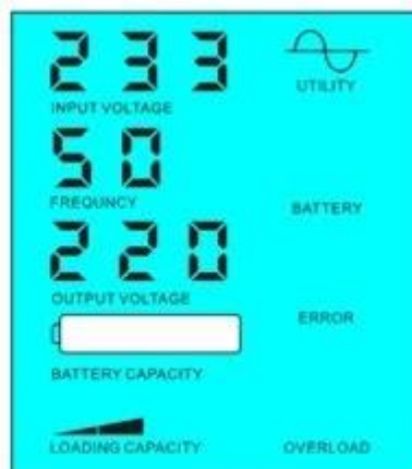
Battery dead, utility supply power
